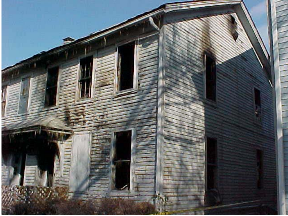
Figure 1. Front of structure. Duplex on right was the unit of fire origin.
